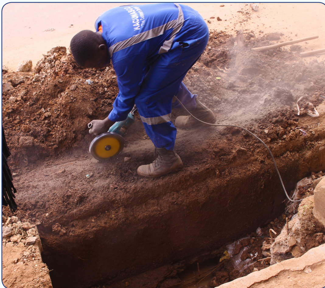
KACWASCO O&M Personnel cut part of the road to access and repair water pipe in Kakamega town
