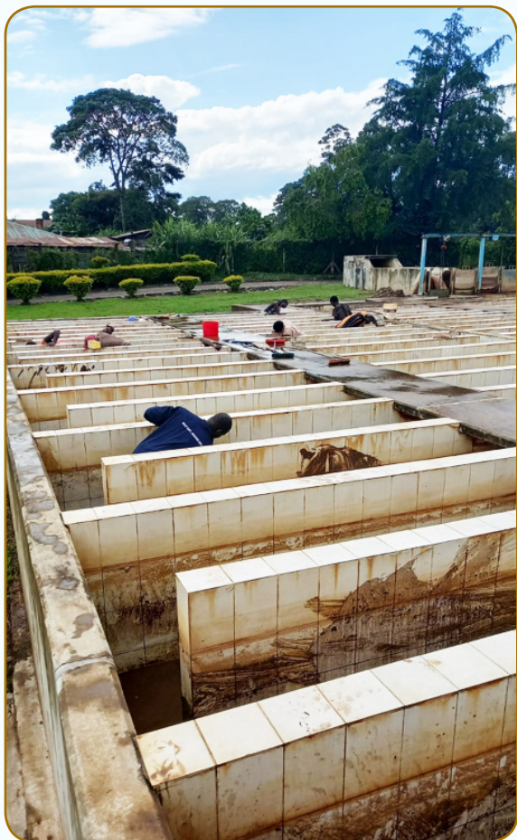
Desludging process at Tindinyo water treatment plant
