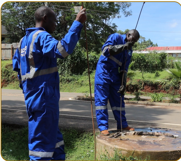
Kakamega Area Waste Water team during routine cleaing of sewer lines in kakamega town
